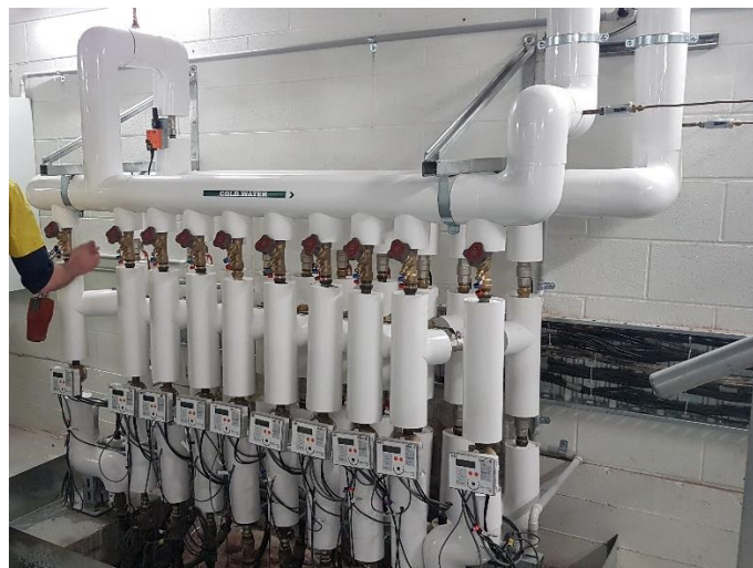
Figure 1: The manifold connecting the heat exchanger U-loops of all the piles.
