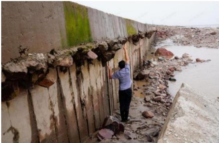
Figure 2. Photo of exposed sheet piles in the south bank scouring seawall.
