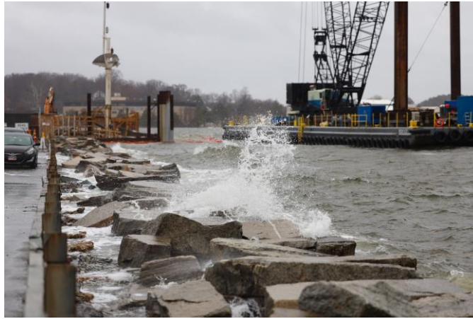
Figure 1. Waves Overtopping Roadway Stabilized by Rip Rap Revetment in Annapolis, MD
