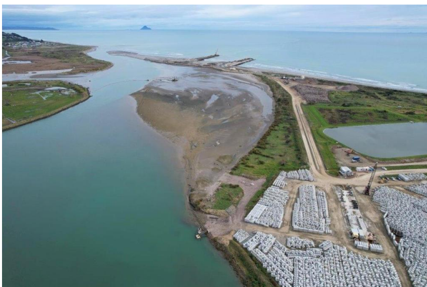
Figure 9. View of Hanbar storage area, dredging, and training walls construction [Source: ODC Government ]
