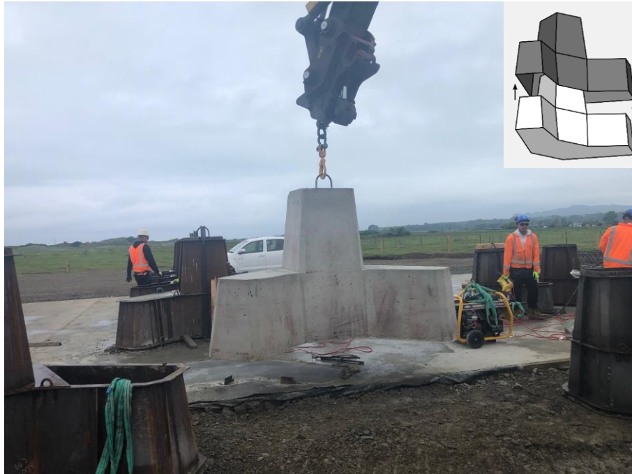
Figure 3. Casting of the first Hanbar unit for the Opotiki project [Source: ODC government ]
