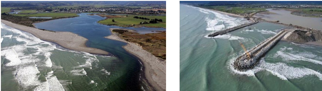
Figure 6. Before (left) and during construction of the entrance works of Opotiki Harbour Development Project
