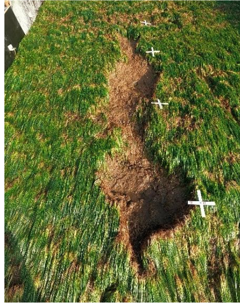
Figure 6 Example of stripped-off turf over roughly 3 m at section 1-1.
