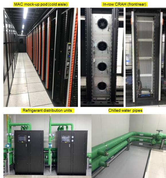
Fig. 3 - A test mock-up system of row-based cooling: sequentially multiple heat exchange system.
