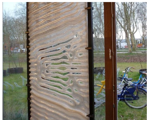
Fig. 13 – Installed full panel of the prototype of the developed PCM based Trombe wall in a meeting room.
