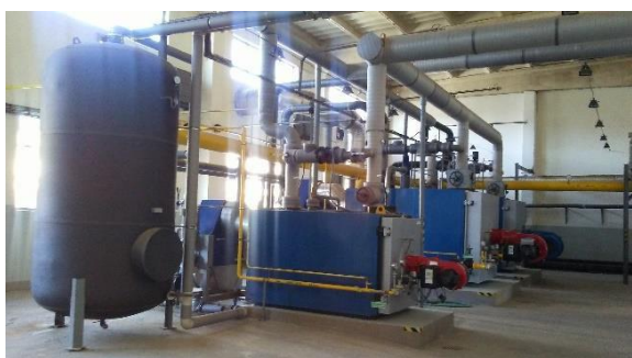
Fig. 1 – Interior view of the existing boiler plant [4].
