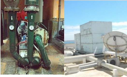
Fig. 1- Old Chiller and Cooling Tower
