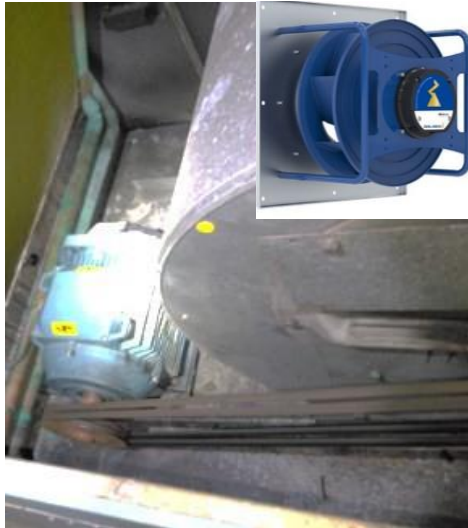
Fig. 12 – Old belt Ventilator and new EC Fan
