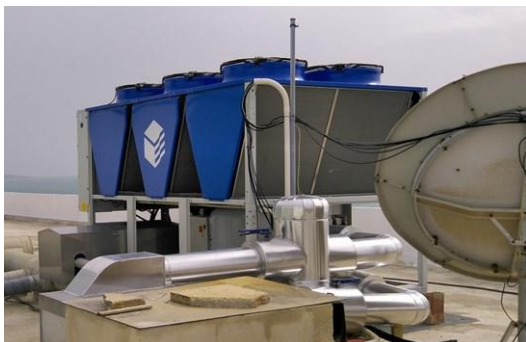
Fig. 8 – New Reversible 2 pipe Chiller 300 kW cooling
