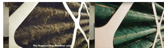
Fig. 1 - Samples of new filter (right) and clogged filter (left), [Theengineeringmindset.com]
