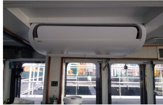
Fig. 2 - Example of additional, separately operated, cooling system in wheel house of one of the smaller ships for day patrols (fan coil unit).
