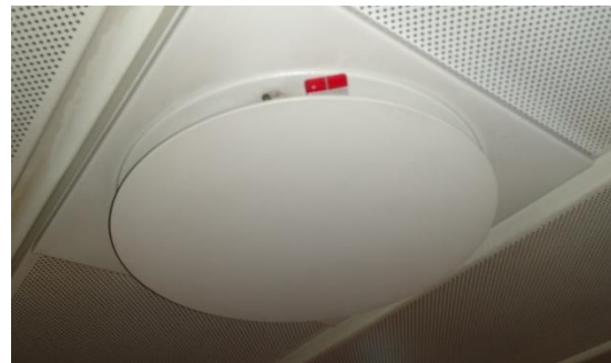
Fig. 3 - Example of supply grill in the mess room of one of the larger ships; note the red handle that can be used to influence the amount of air supply.
