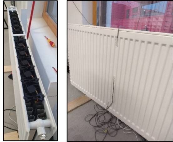
Fig. 4 – Array of fans with the covering grille removed (left) and view of cooling radiator (right).
