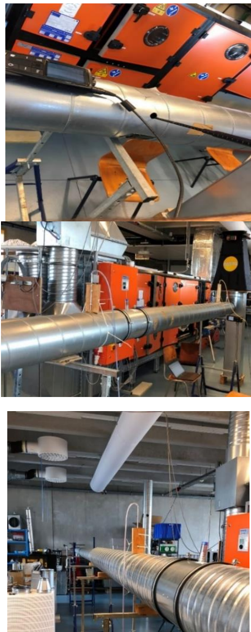
Fig. 3 - Experimental setup – UAntwerpen HVAC Lab
