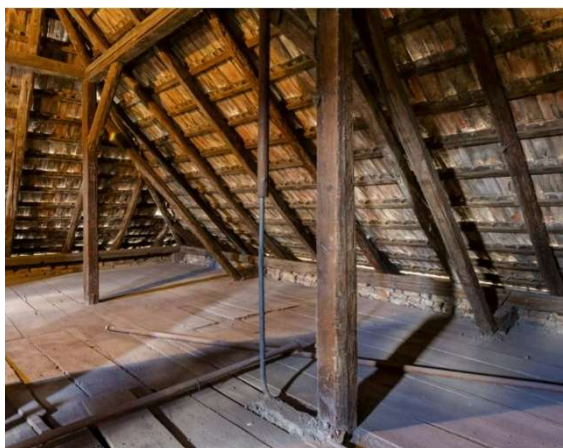
Fig. 7 - The old degraded wooden truss before renovation of the house [2, 3, 4].
